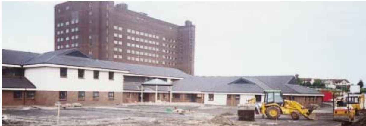
THE NEW LARKFIELD UNIT FOR ARGYLL & CLYDE ACUTE HOSPITALS NHS TRUST IS NEARING COMPLETION. BUILT IN THE GROUNDS OF INVERCLYDE ROYAL HOSPITAL, THE NEW UNIT WILL HOUSE 120 GERIATRIC BEDS.
